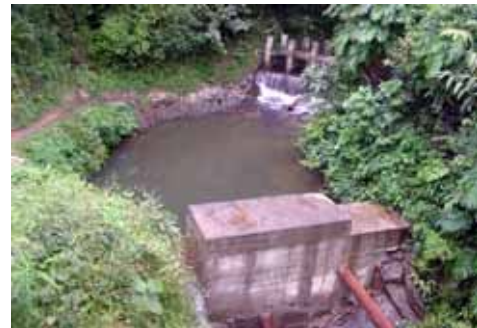
Fore bay tank and diversion weir
